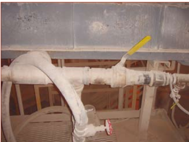
Figure 7. A tie-in between the low-pressure and high-pressure systems.
