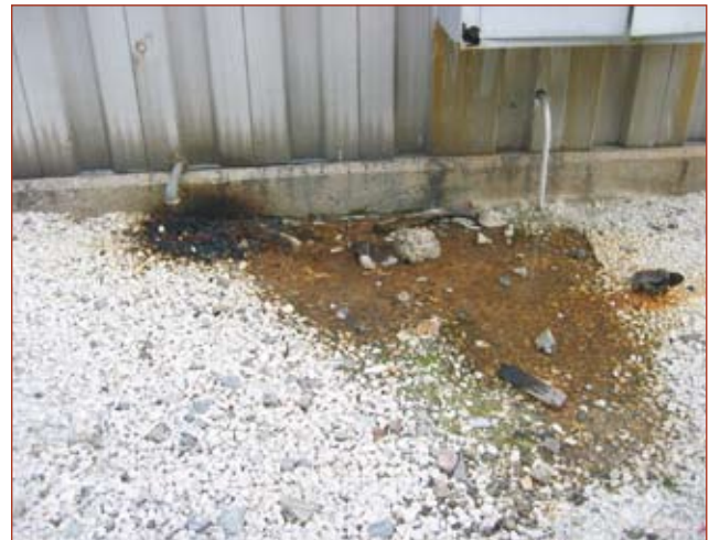
Figure 11. Condensate containing water and compressor oil draining onto the ground.
