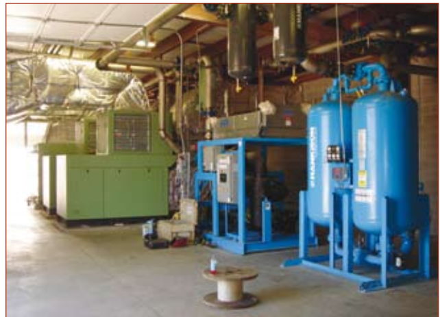
Figure 8. Heat recovery for a compressor room.
