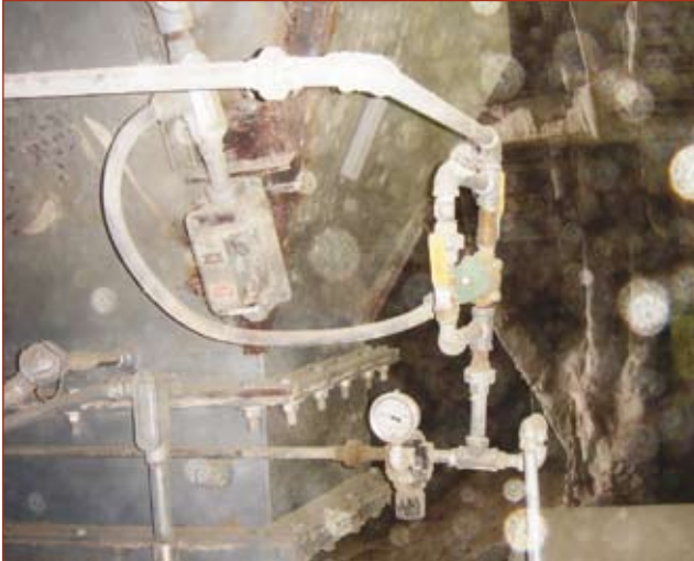
Figure 5. Another FK pump example where an off pump consumed air since the solenoid was bypassed.
